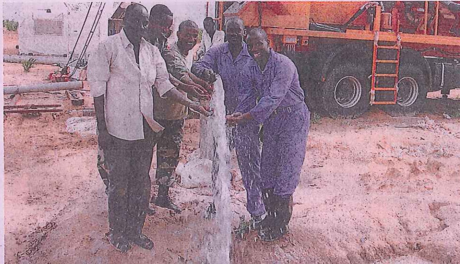
Water flows from a new well sunk by one of the three Dando drilling rigs now in use by a United Nations organisation working in Darfur, Sudan.
