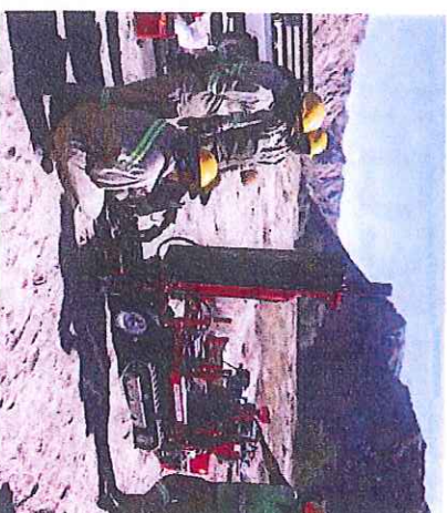
April, the Terrier successfully took core samples from 21.9m deep - bordering on the mini multipurpose rig's maximum drilling capacity with the diameter and geology in mind.
